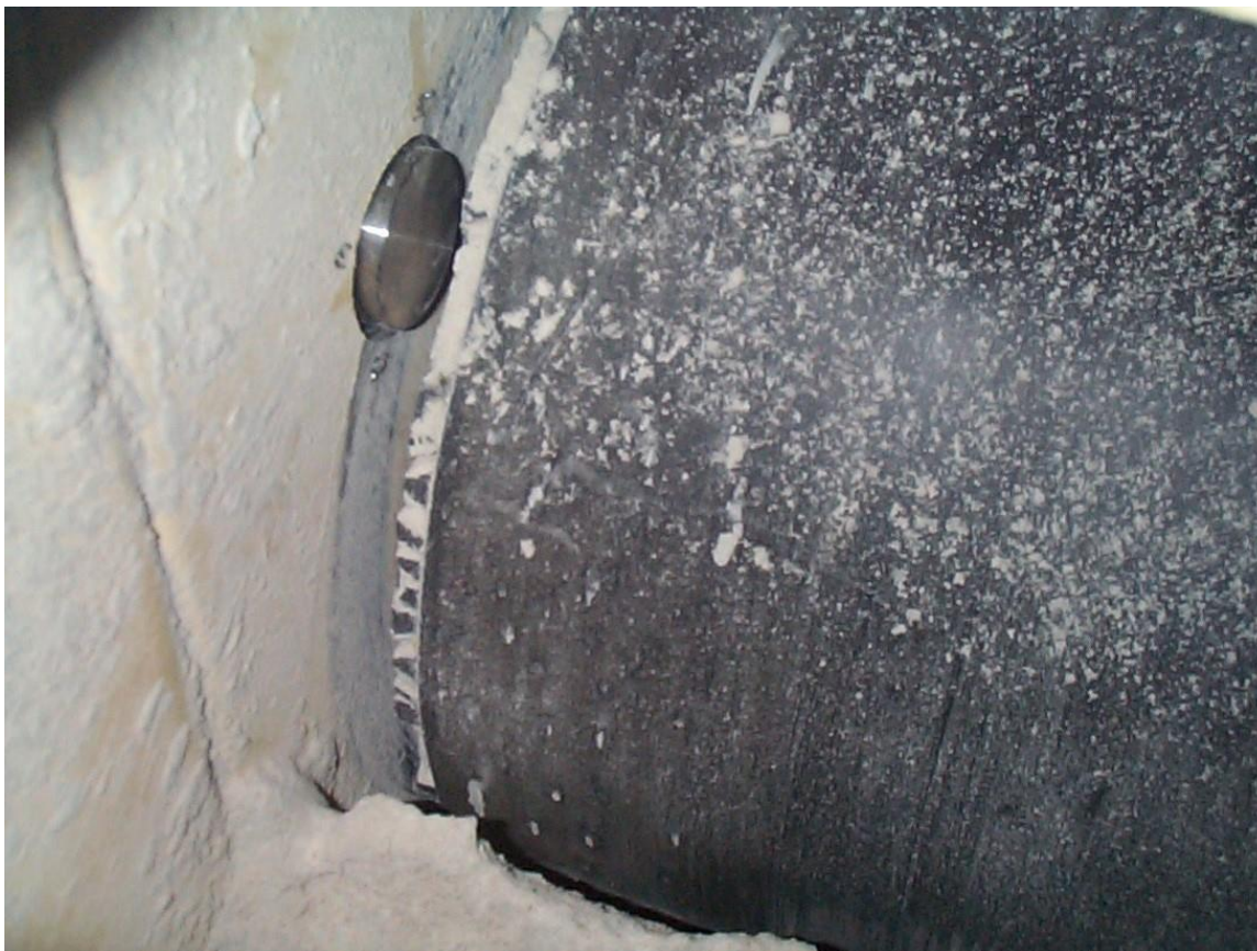
Figure 21: Interior view of belt conveyor head with misalignment sensor monitoring both belt and pulley. (Photograph courtesy of 4B Components, Ltd)
