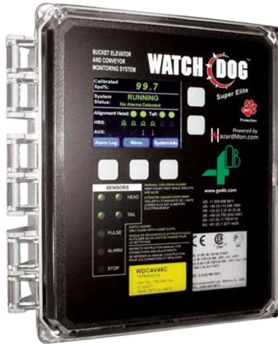
Figure 31. Typical single conveyor hazard monitoring system. (Photograph courtesy of 4B Components, Ltd.)
