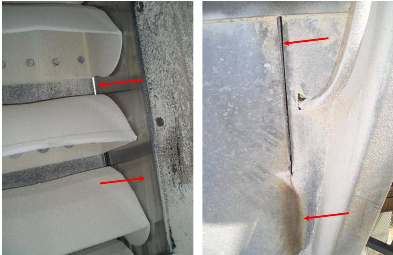
Figure 16: Inside elevator (left) and outside elevator (right) showing discoloration and slits in steel casing from the effects of friction and wear due to severe belt misalignment. (Photographs courtesy of 4B Components, Ltd)
