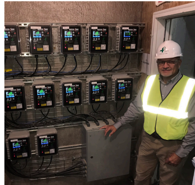
Several Watchdog Super Elite and Flex-Net Industrial Ethernet Systems installed in a facility control room
